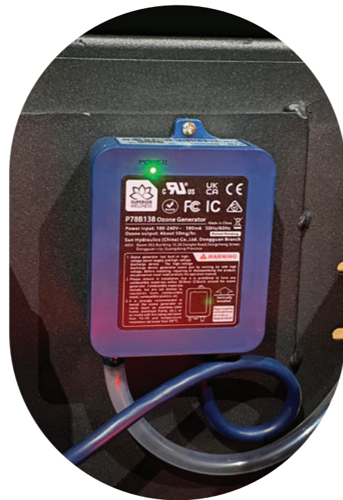
Ozone and Filtration systems
